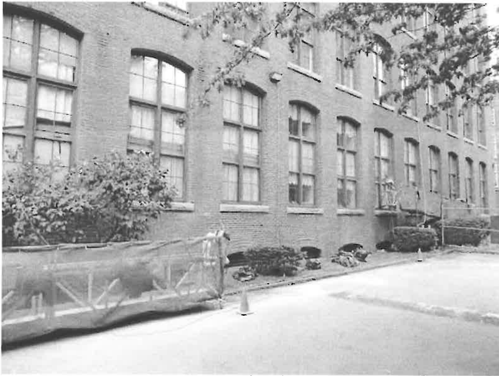
Photograph 1 – Staging at the bottom of the 3 rd & 6 th drops to be moved to the last two drops.
