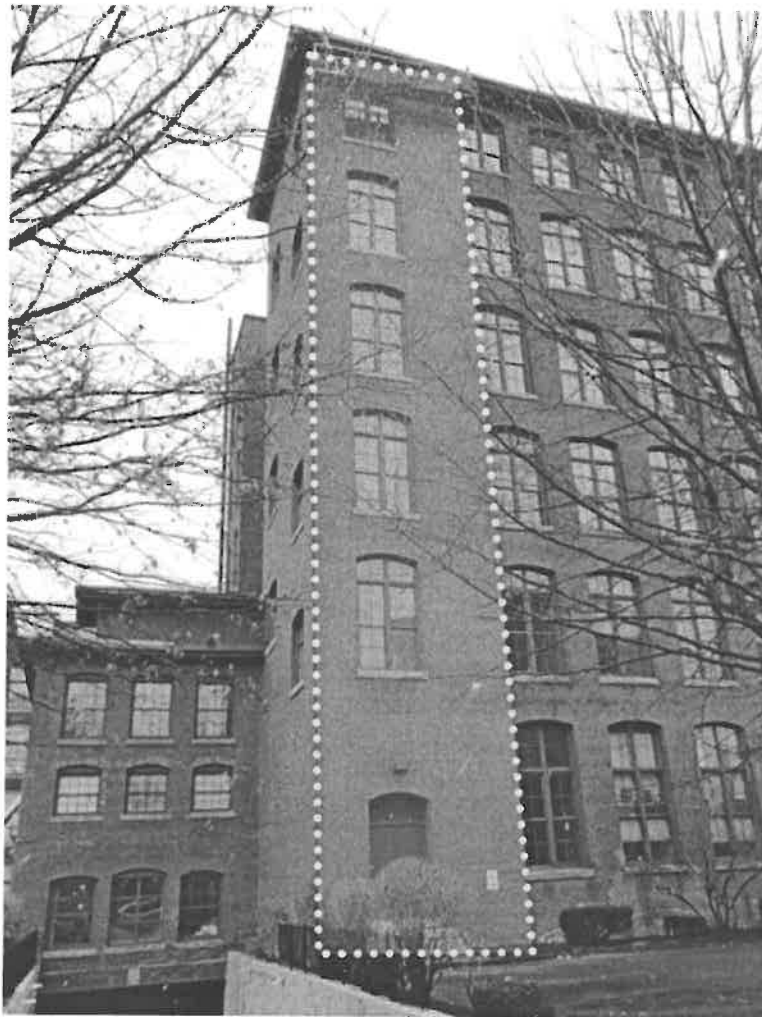
Photograph 1 – Cutting and pointing of masonry on the north elevation in the highlighted area is complete.
